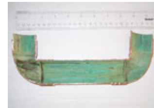
Cut-away of copper pipe showing blue green corrosion.
