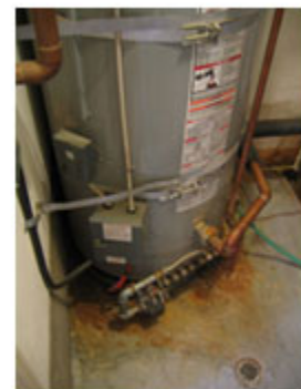
Corroded leaking water heater caused by acid water corrosion.
