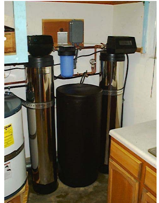
Sediment backwash filter followed by 1 micron filter and water softener. Removes sediment, iron and softens water.
